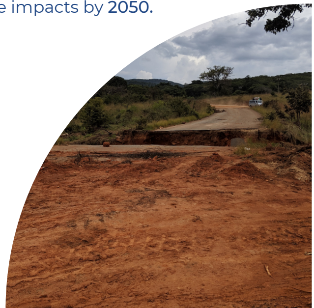
Result of landslides and flooding in Zimbabwe.
